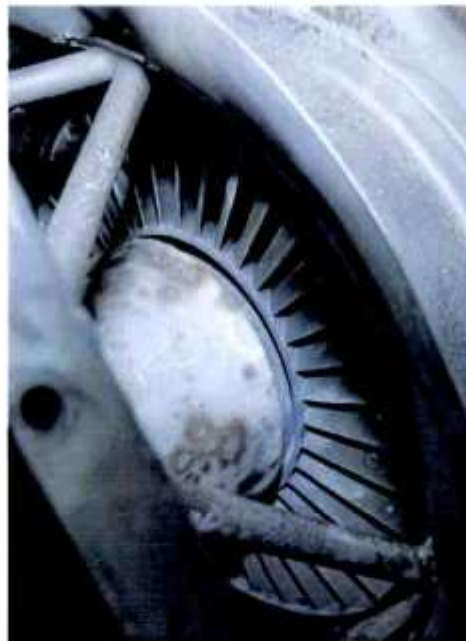
Photo 3 Fourth Stage Turbine Wheel
