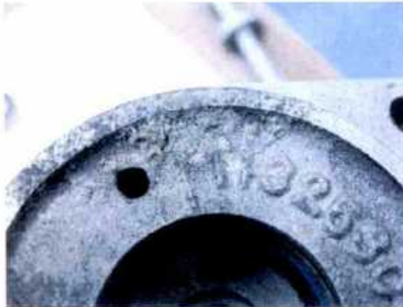
Figure AI-13: Pump mounting face (corrosion product)
