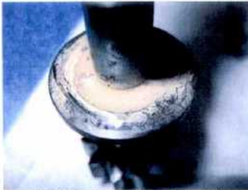
Figure AI-25: Main drive shaft (corrosion product)
