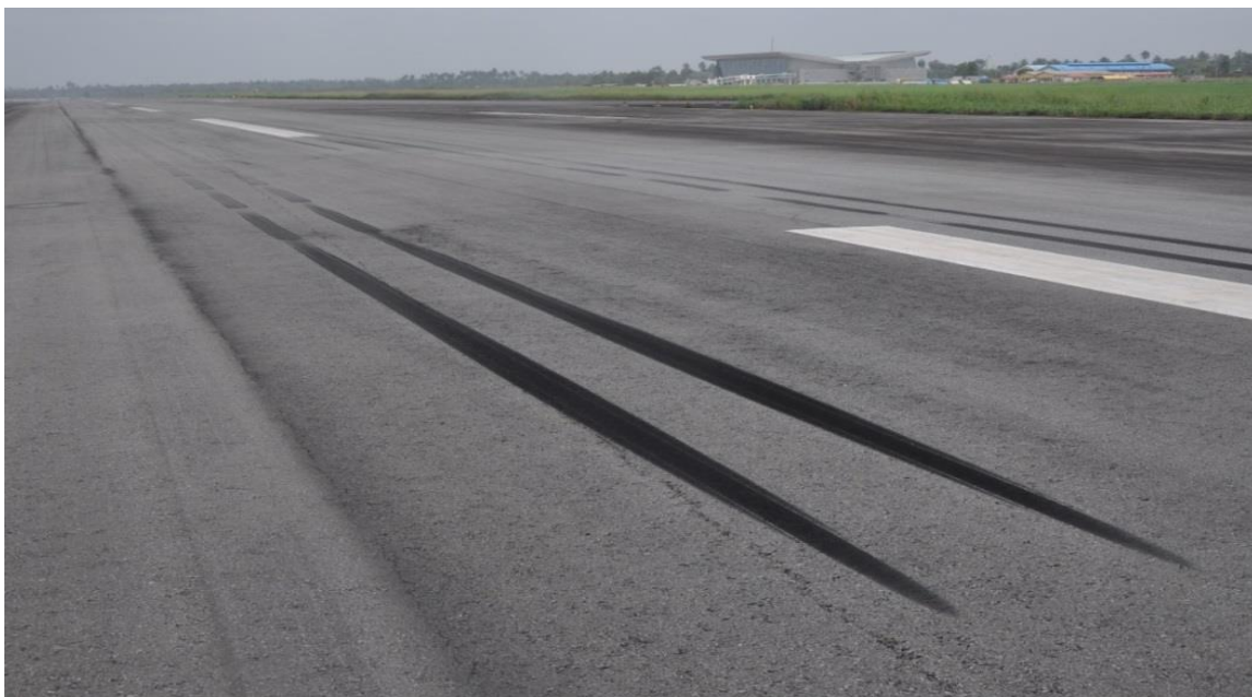
Figure 4: Tyre marks from the right main landing gear of the aircraft
